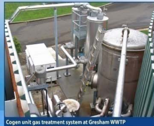
Cogen unit gas treatment system at Gresham WWTP
